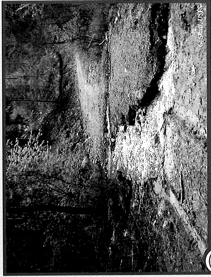
Poorly designed and maintained roads can alter watershed hydrology and degrade water quality.
